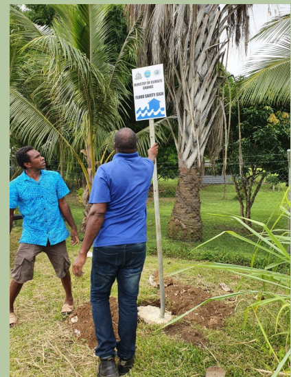
Installation of Flood Safety Signage for Teouma Bridge Community and Salili Bridge Community
